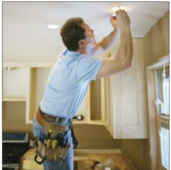
Be careful not to install new lighting to old, inferior wires. To avoid this fire hazard, check your wire rating first and either upgrade it or buy fixtures within the supply connection range. Photograph courtesy of Electrical Safety Foundation International
